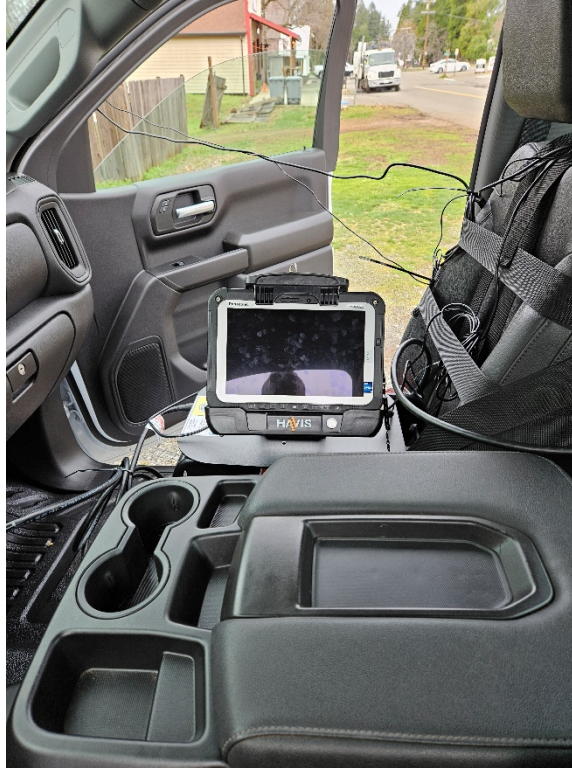
Automatic meter reading equipment installed in vehicle
